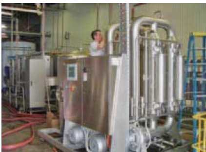
Installation of 200sqm ceramic crossflow filter at Loxton.
